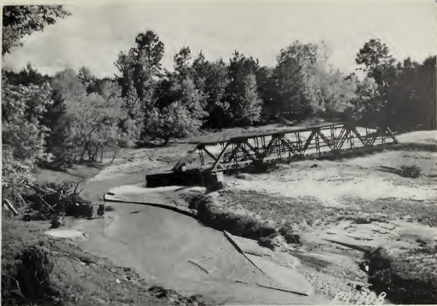
Destruction precipitated by products of erosion. This stream channel has silted up to the bridge level, leaving the bridge "high and dry" and useless.
